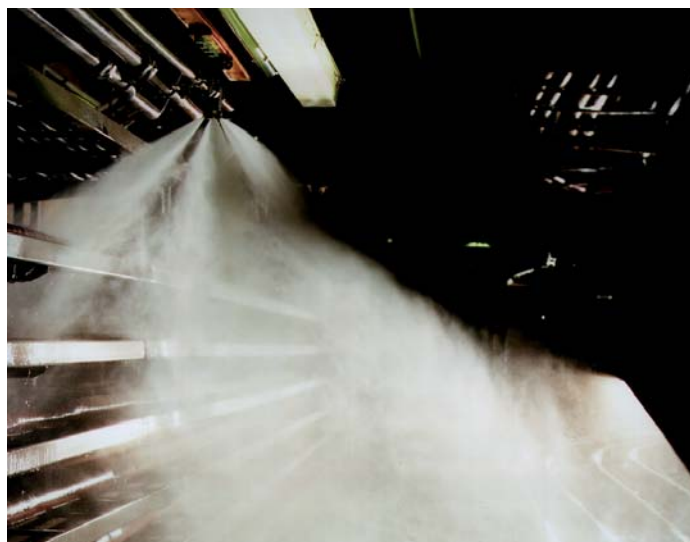
Fig. 5: Triggering of the water-mist system in a cable duct (source: FOGTEC)
